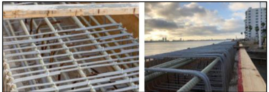
Pictures of MST-BAR® being used on a seawall project in Florida – images from TUF-N-LITE website
