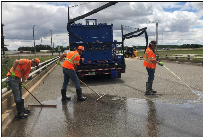
Workers applying and spreading E-TUFF® 7097 on a bridge deck – image from PSI
