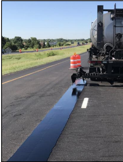
J-Band Longitudinal Joint Sealer being applied – image from Asphalt Materials, Inc. brochure
