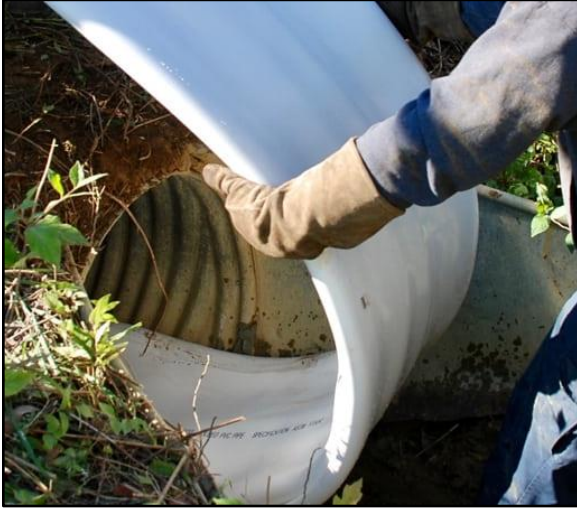
Worker pulling the Warrior Thermoform pip-liner through a metal pipe – image from Thermoform Website
