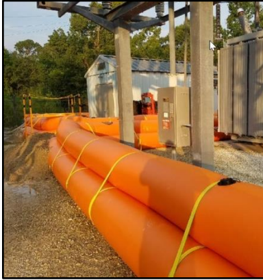
Tiger Dam™ protecting an electrical substation prior to flooding – image from U.S. Flood Control Website
