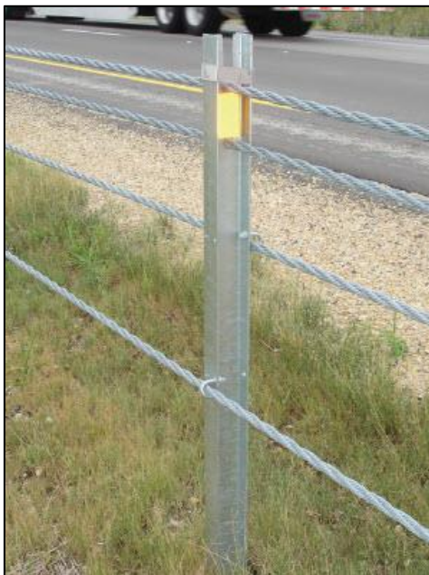
CASS® S3 M10 TL-3 and TL-4 median cable barrier system installed along a highway median - image from Trinity website
