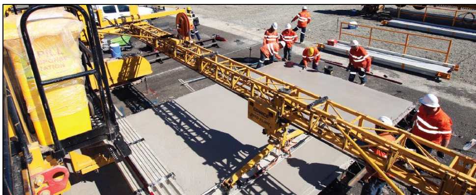
Workers using a slip-form paver to install Geopolymer EFC ™ at an airport in Australia – image from PGM brochure
