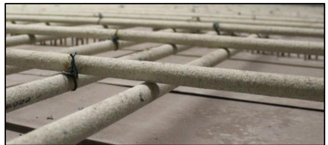
Grey/white BFRP rebar tied together prior to a concrete pour for a parking garage floor – image from Pultrall twitter account
