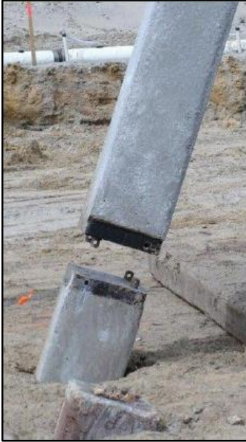
Two concrete piles with an EMECA Splice on each end about to be joined in the field - image from EMECA/SPE USA Brochure
