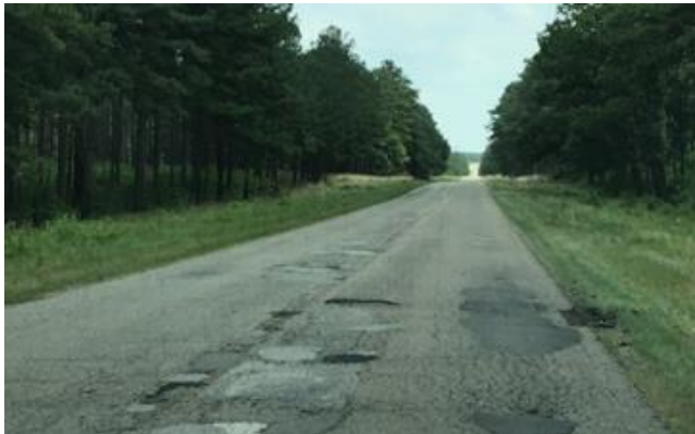
Figure 2 – Pavement Condition along King Road
