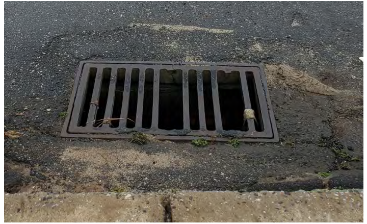
Existing drainage infrastructure in need of improvement
