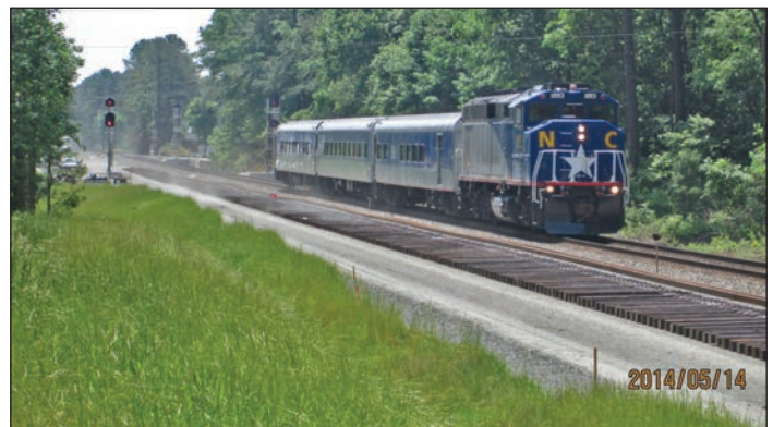
The Piedmont passes through the second track construction work zone of U-4716 Nelson to Clegg at McCrimmon Parkway.
