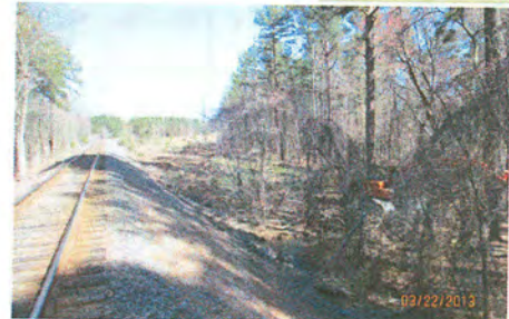
P17 & P18-Hopson/Clegg: This project is located between MP H-63.6 and H-67.0 on the NCR/NS H-line near Morrisville, North Carolina, and is to be completed in conjunction with Project P17: Clegg to Nelson Passing Siding.
