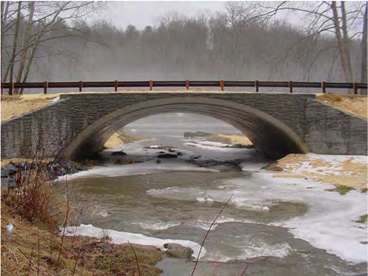
Figure 4: The stone arch look of the completed project was achieved by using concrete formliners. Due to low temperatures, the concrete stain has not yet been applied.
