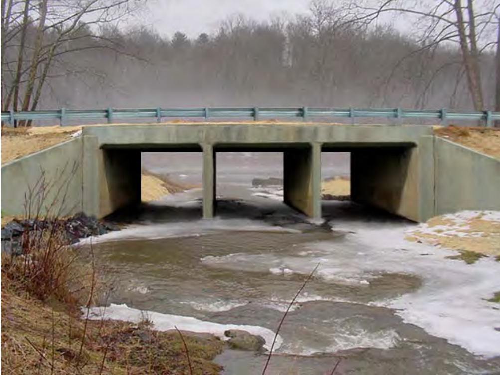
Figure 2: A computer visualization of the project utilizing a triple 12' X 9' RCBC. This option was derided by the community as being visually unappealing.
