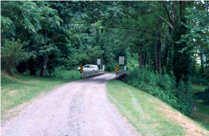
Figure 1: The old Grassy Creek Bridge carried a one-lane gravel road with a clear roadway width of just over 11 feet.
