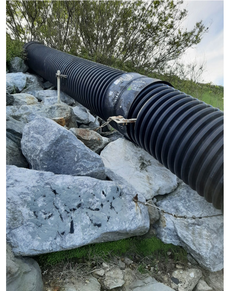
Note: Photo is shown for dramatization purposes. Pipes must be buried.
