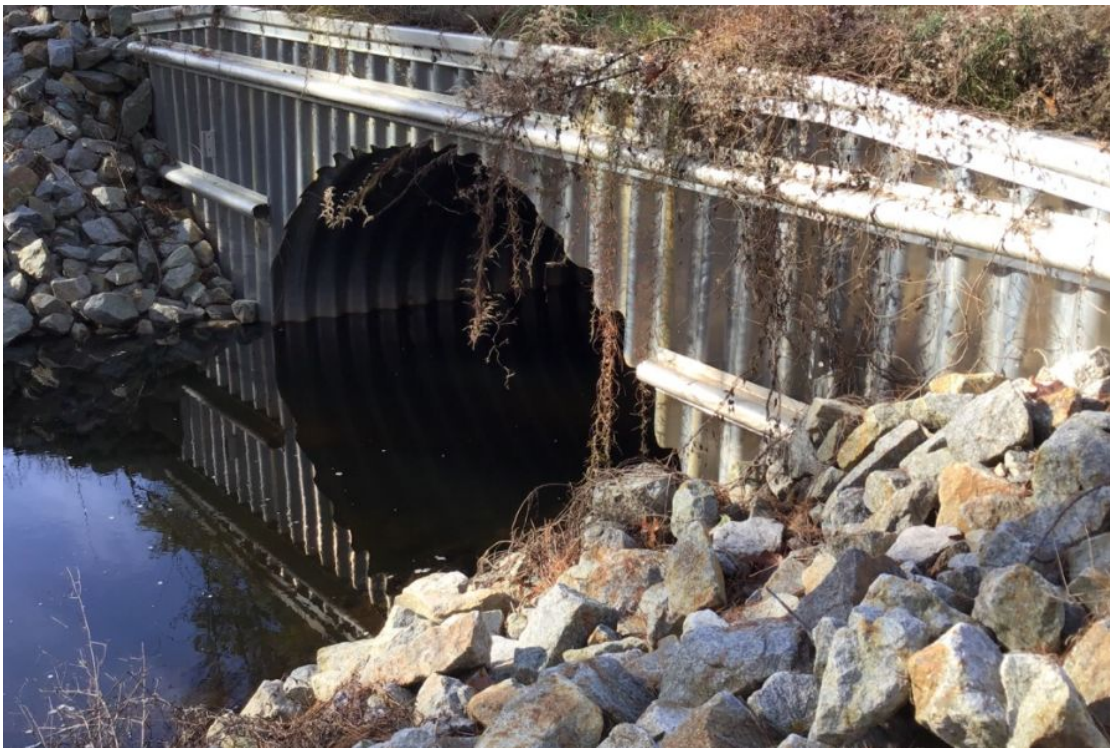
Corrugated Metal Headwall for CMPA
