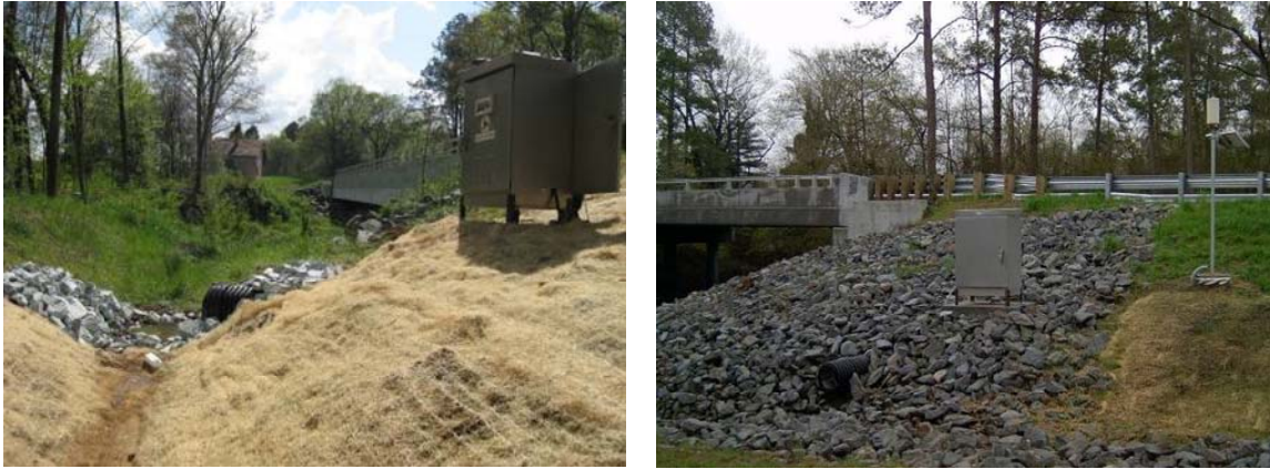
Figure 3.2-2: USGS bridge deck runoff monitoring equipment: bridge deck runoff monitoring box and modified outlet pipe at Mountain Creek (left) and monitoring equipment, including a rain gage, at Black River (right).
