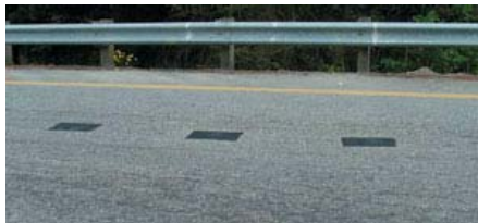
Electromagnetic sensors embedded in the pavement (the three dark squares) detect vehicles moving in the wrong direction.
