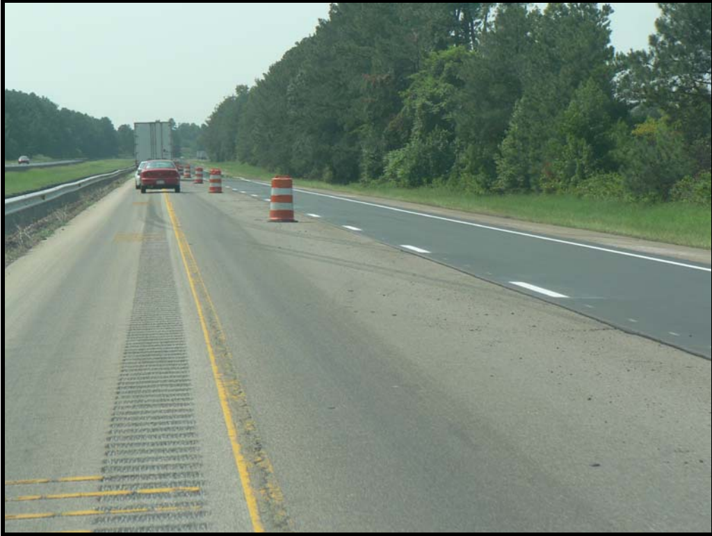
Squeezing of Traffic, Riding on Rubble Strips near WZ Workers
