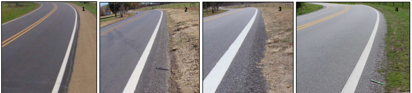
SR 1007 in Johnston County (1) initially after the shoulders were pulled, and at (2) 13 months, (3) 19 months, and (4) 37 months after resurfacing.
