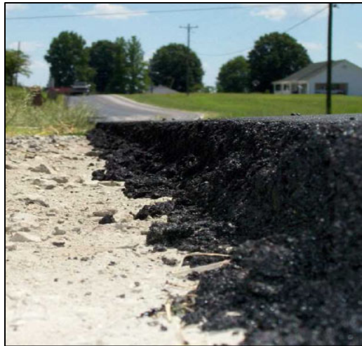
SR 1611 in Burke County: Resurfacing Without Safety Edge
