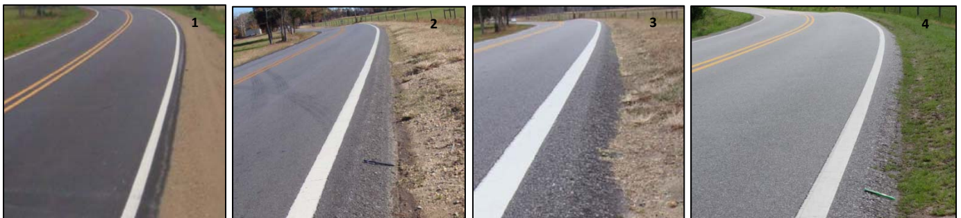
SR 1007 in Johnston County (1) initially after the shoulders were pulled, and at (2) 13 months, (3) 19 months, and (4) 37 months after resurfacing.
