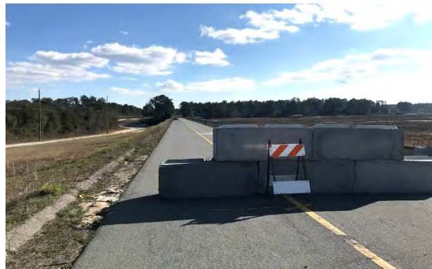
Collapsed Sanford Dam on Alton Lennon Road
