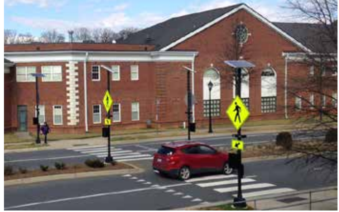
Pedestrian crossing signals installed between two schools in Davidson, NC.
