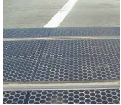
Installing a rubber surface rather than asphalt around railroad flangways reduces changes in level and other maintenance problems.
