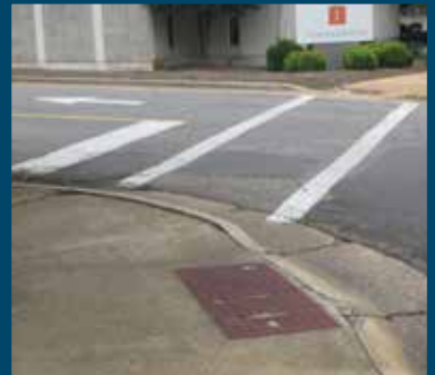
Crosswalk markings do not line up with curb cuts/ ramps:
