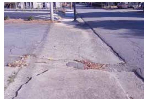
Crumbling sidewalks are a regular scene around many parts of Newton
