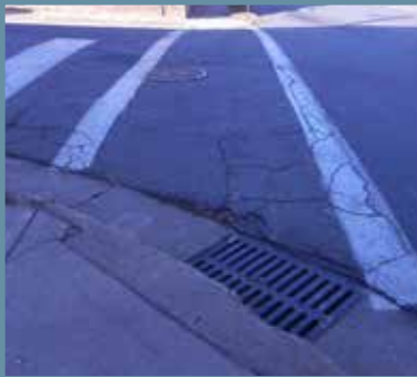
Sewer grate in crosswalk- unsafe for wheel chairs, strollers, bicycles, etc.:
