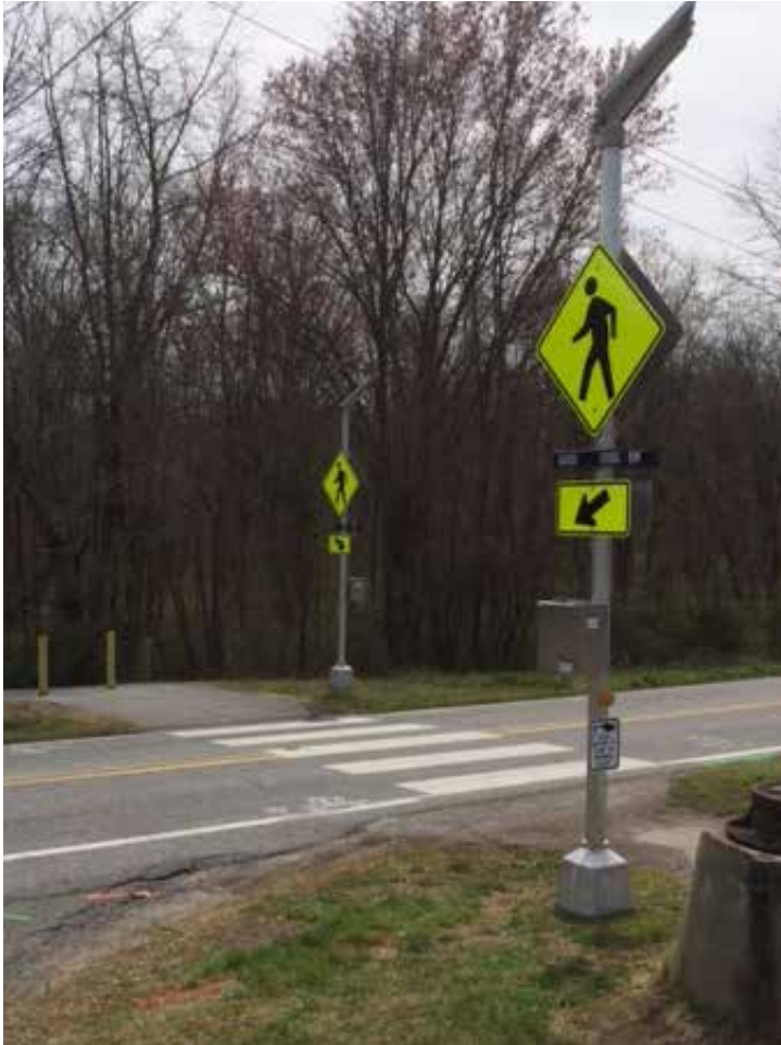
This RRFB was installed in March 2017 at the Radio Station Road crossing of the Heritage Trail Greenway
