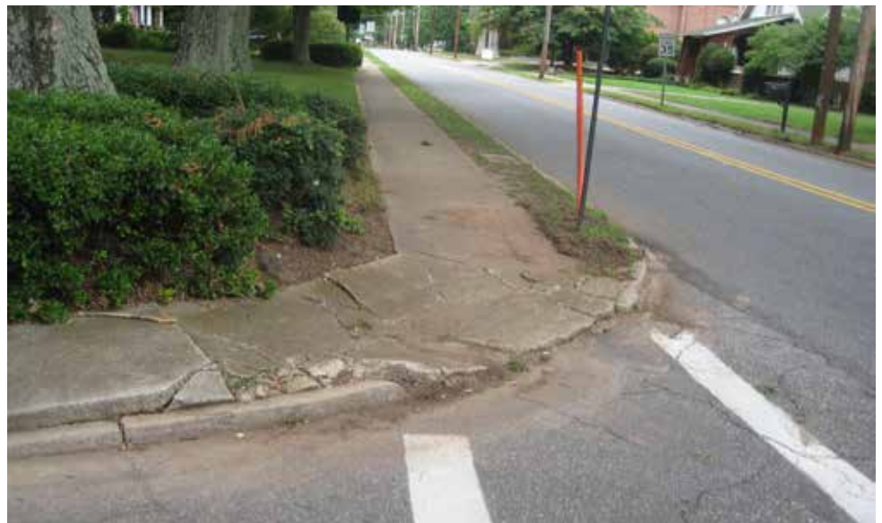
Crumbling sidewalk at intersection of North Main Avenue and West 6th Street.
