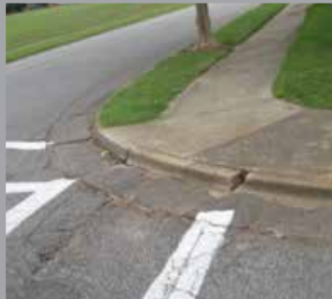
No curb cut at crosswalk:
