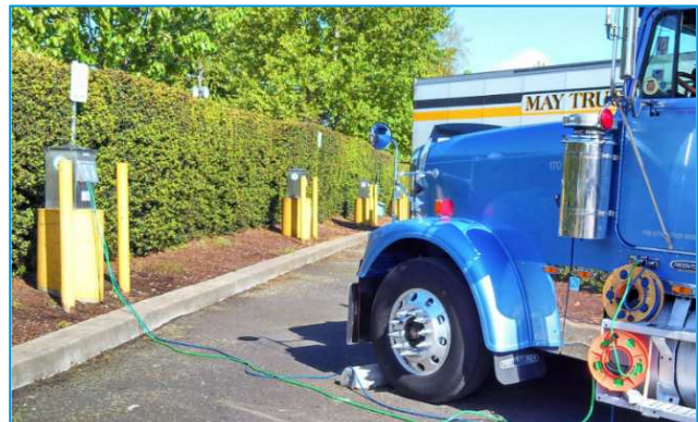
Truck Stop Electrification
