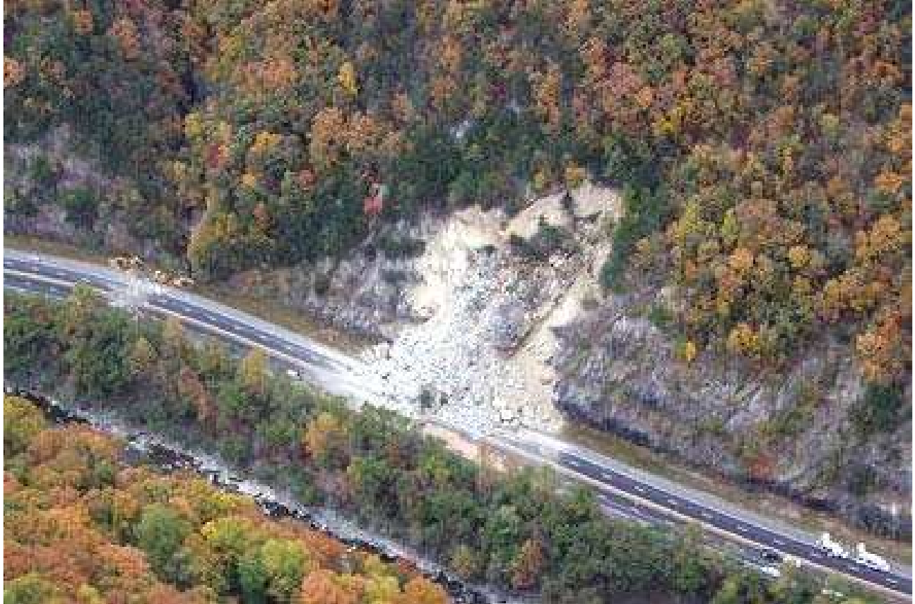
Figure 3.8 February 2019 Rockslide Damage I-40
