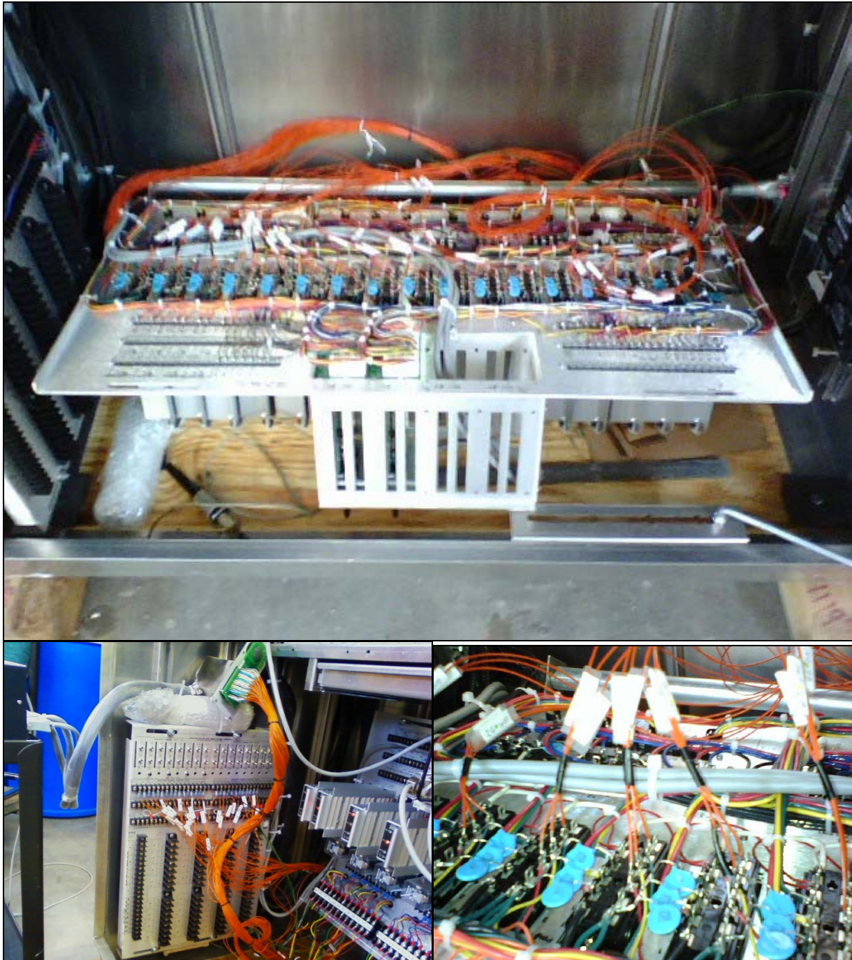
Figure 4.17 Soldered Connections of the Individual Wires from the 170 Cable to the 2070-2A Field I/O Module in the TS-2 Cabinet
