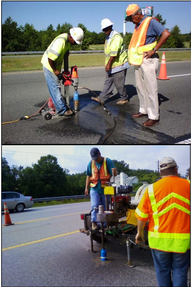
Figure 4.22 Installing the Wireless Sensors in the Pavement at US 70 and Swift Creek (left) and NC 280 and Ray Hill Road (right)
