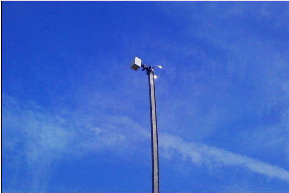
Figure 4.25 A Repeater Installed Atop a Temporary Pole Adjacent to the Detectors
