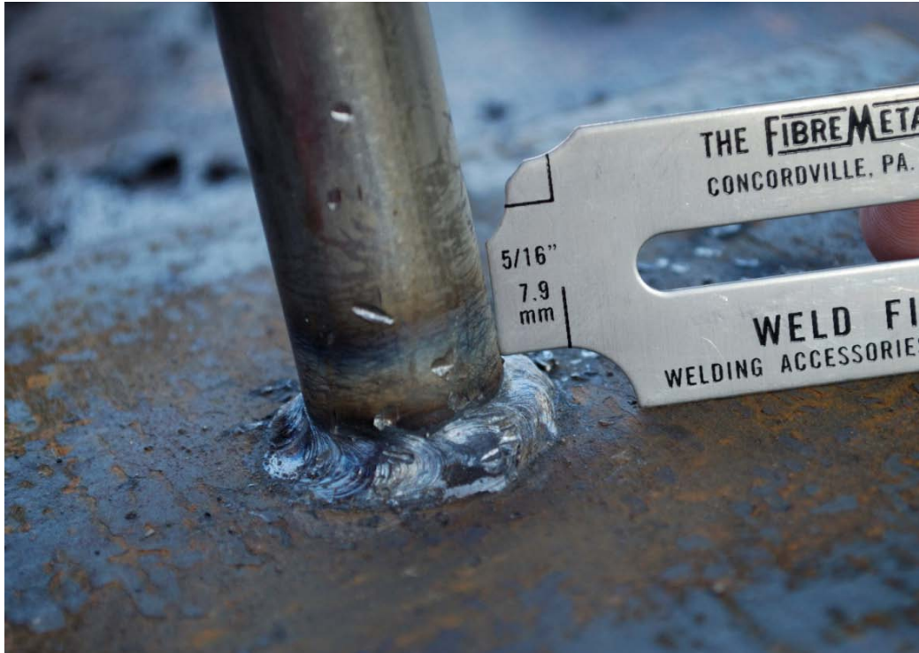
Unacceptable weld (too small)
