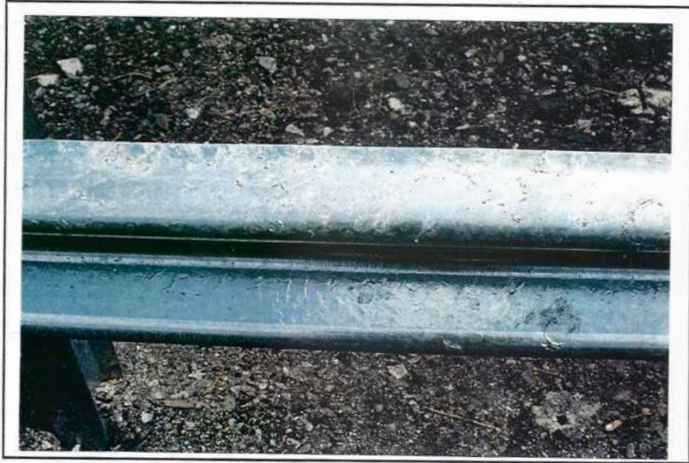
Photo 48 Condition: Ash Inclusions
