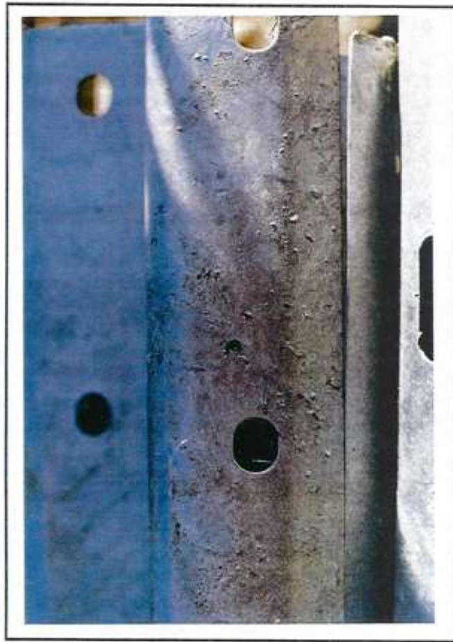
Photo 54 Condition: Ash Inclusion
