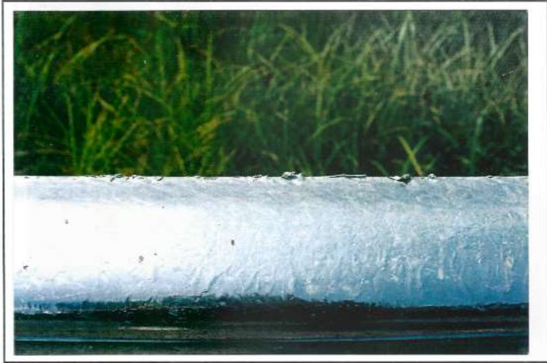
Photo 21 Condition: Excess Buildup of Material
