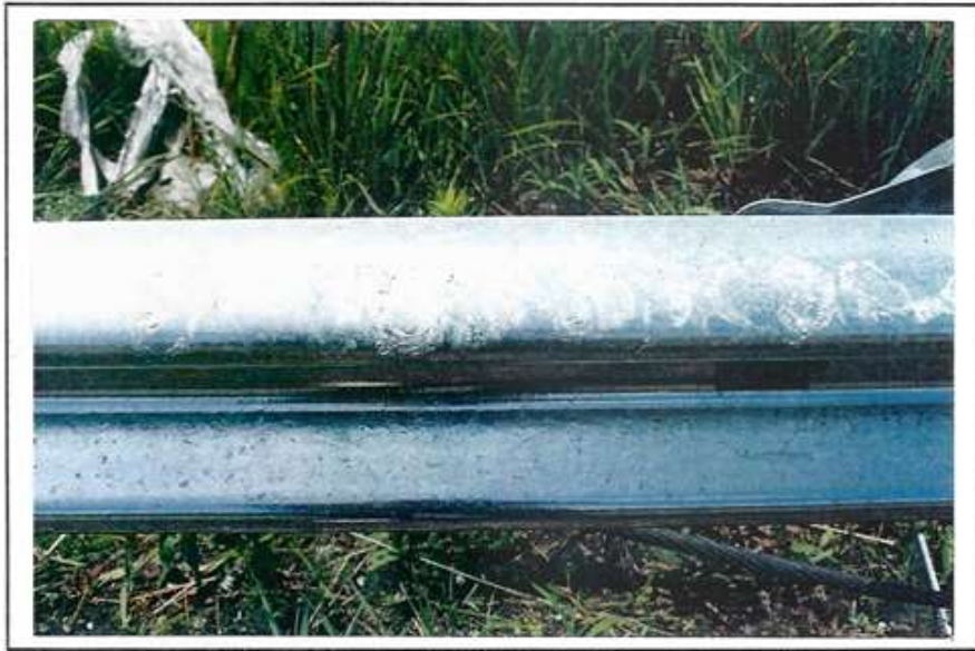
Photo 55 Condition: Ash Inclusion
