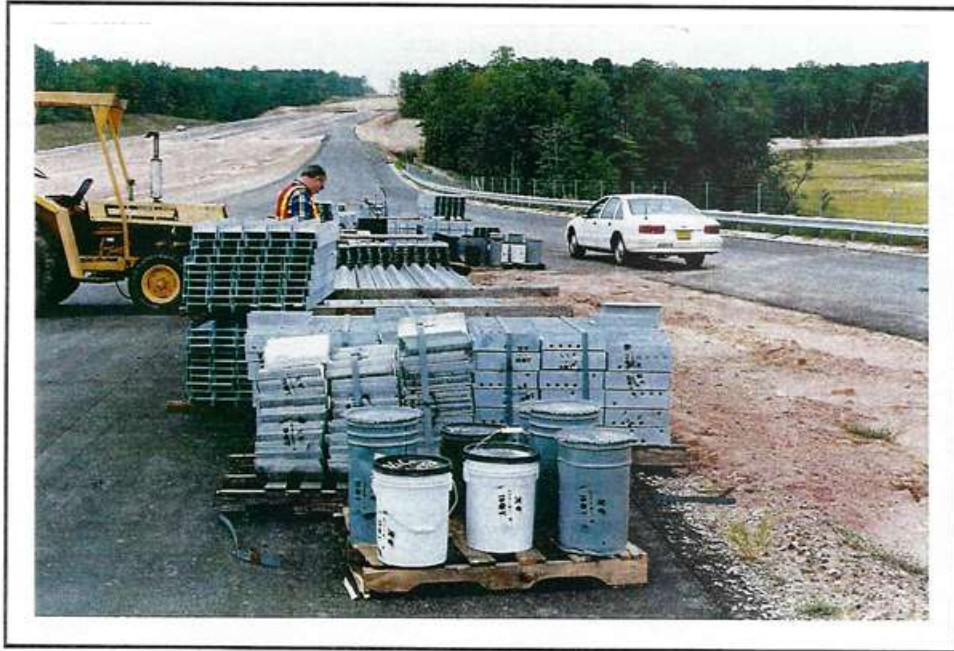
Photo 87 Proper storage of guardrail material. All materials are placed on pallets and all containers have lids.
