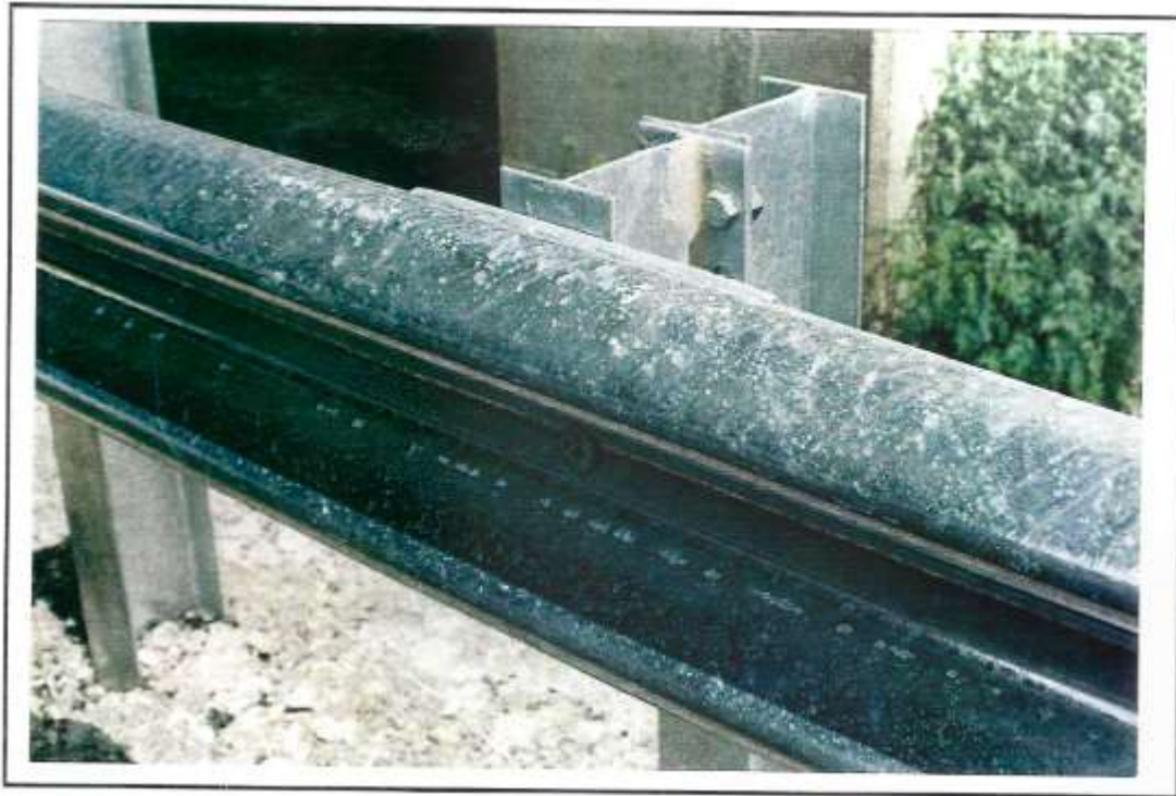
Photo 28 Condition: Dull Gray Coating or Mottled Appearance
