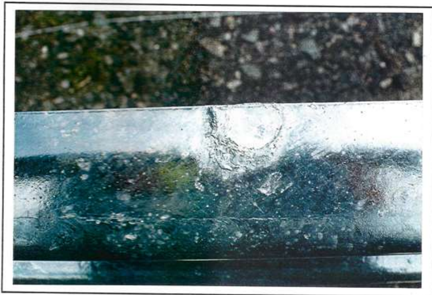
Photo 50 Condition: Ash Inclusions
