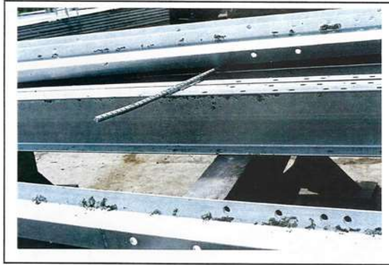
Photo 43 Condition: Bare Spot
