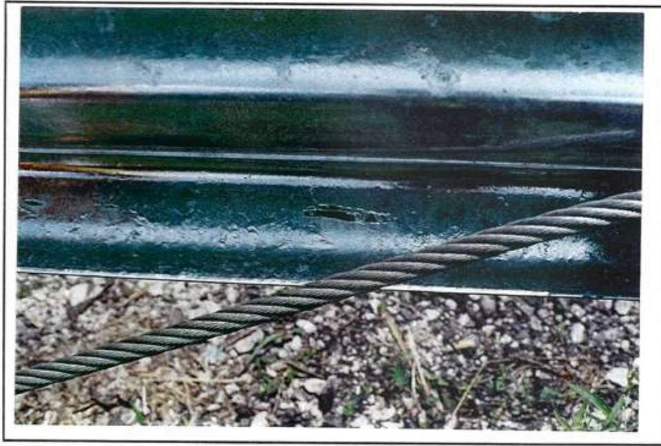
Photo 42 Condition: Bare Spot
