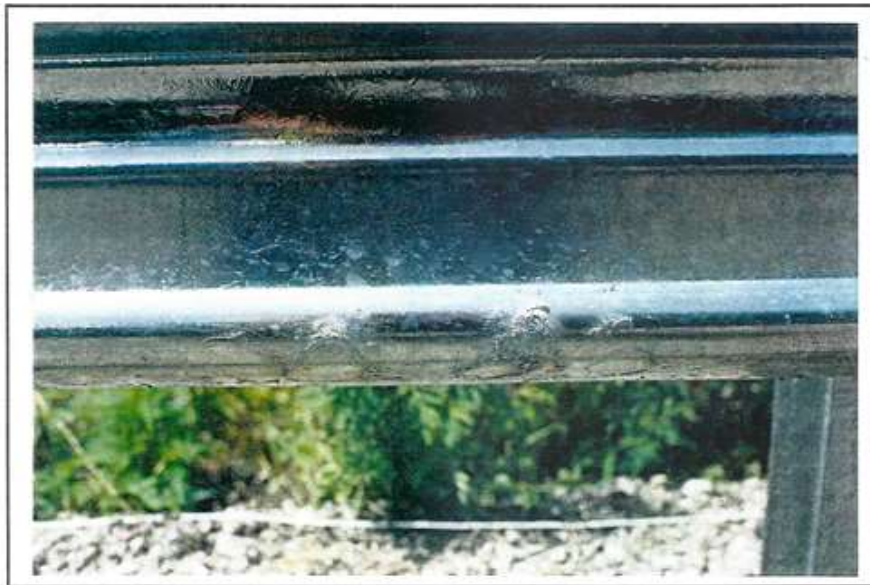
Photo 56 Condition: Ash Inclusion
