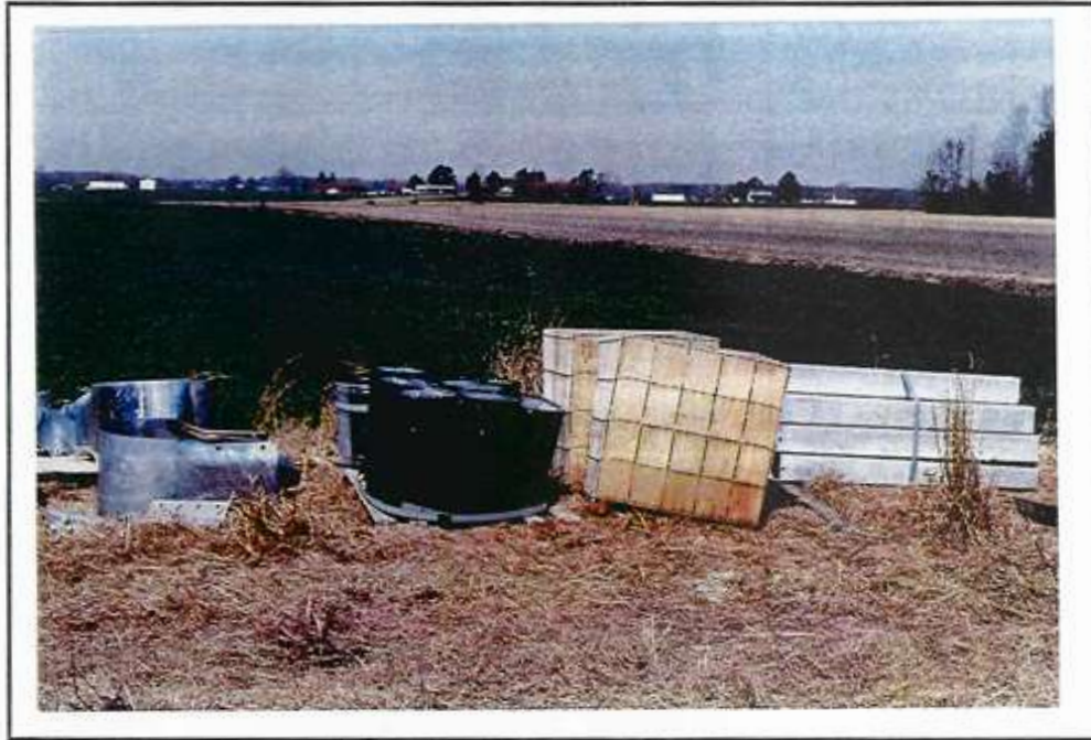
Photo 82 Improper storage. Material is in contact with decaying matter and the ground surface.
