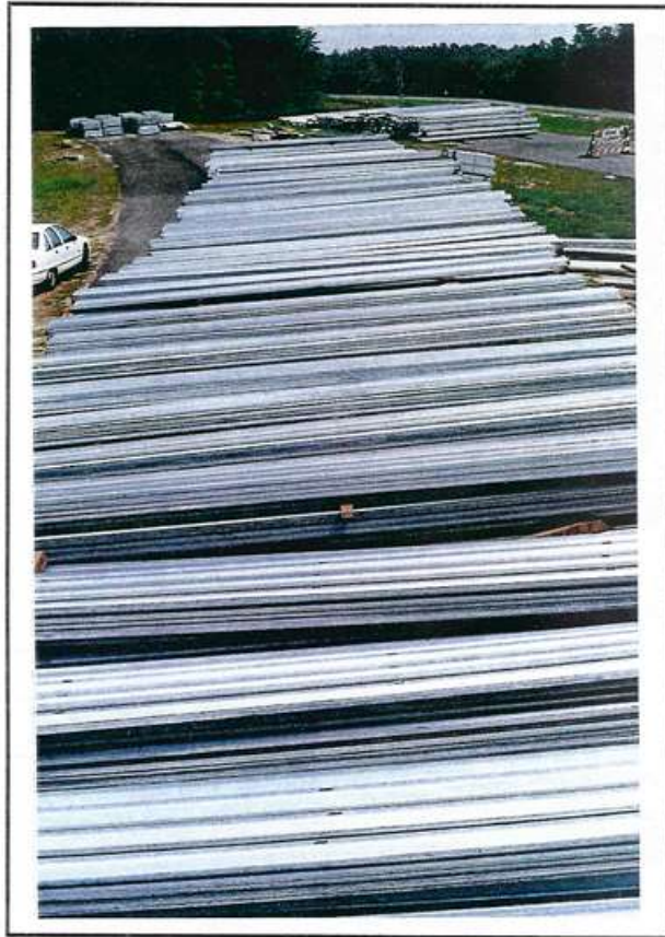
Photo 79 Materials stored at construction site. The rail is slanted to aid in moisture runoff. However, if the material is to be stored for over one month, it should be covered.
