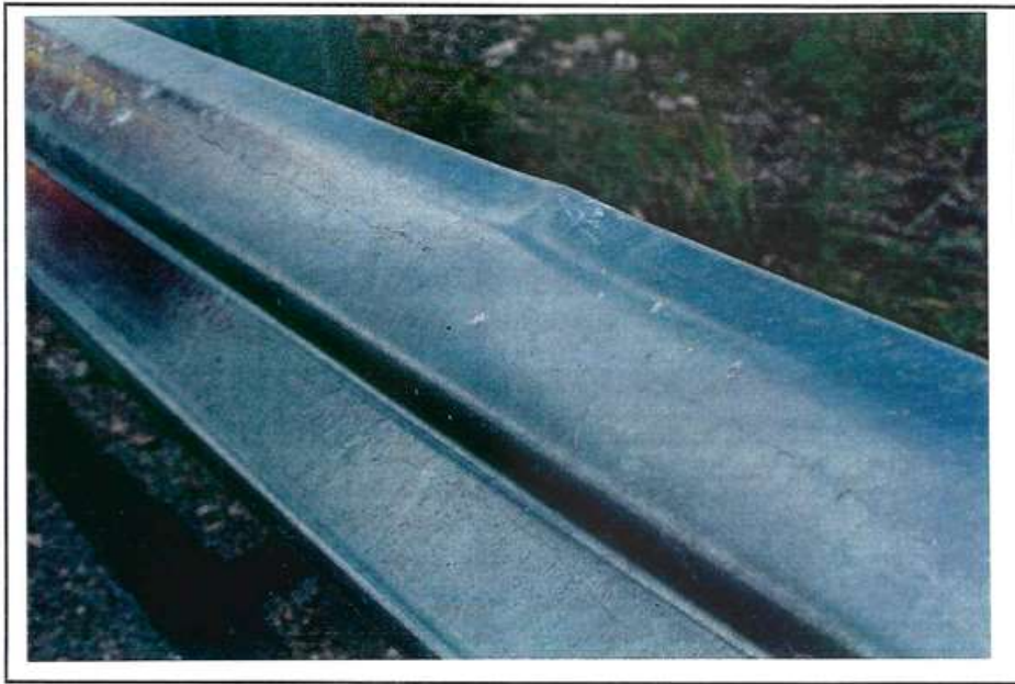
Photo 59 Condition: Bent Rail (Cracked or Broken Galvanization)
