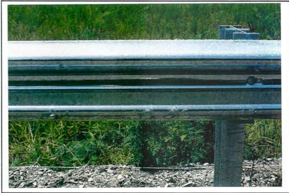
Photo 57 Condition: Ash Inclusion
