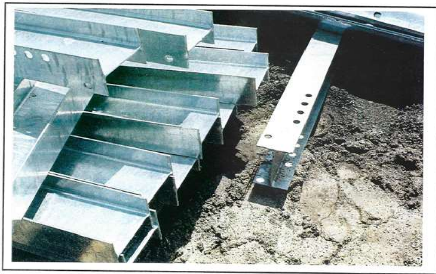
Photo 81 Improper storage. Galvanized material should not be exposed to or stored in contact with the ground surface.
