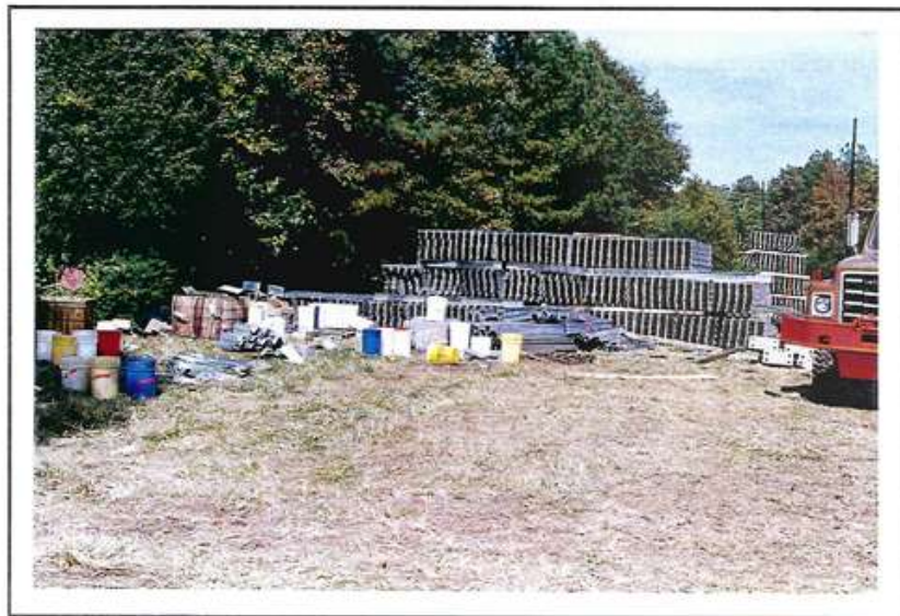
Photo 85 Improper storage. None of the containers have lids on them to keep rainwater or other moisture from getting into containers. Additionally, materials are stored in contact with the ground surface.
