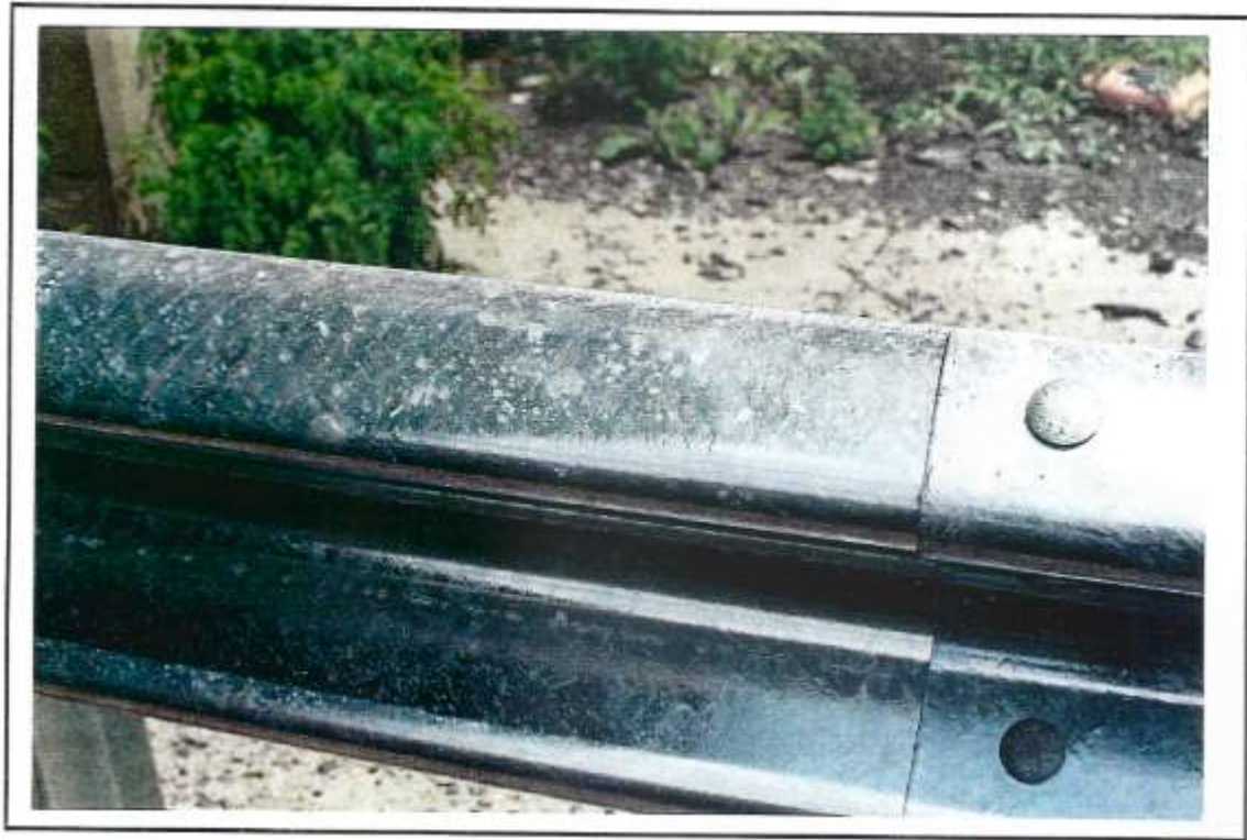
Photo 27 Condition: Dull Gray Coating or Mottled Appearance
