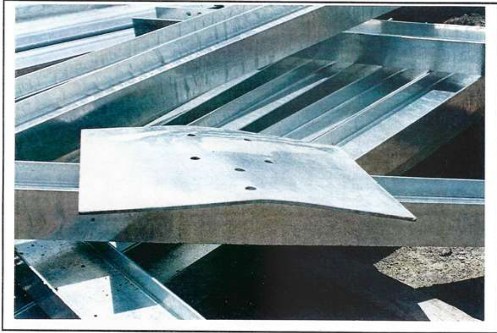
Photo 63 Condition: Bent Plate
