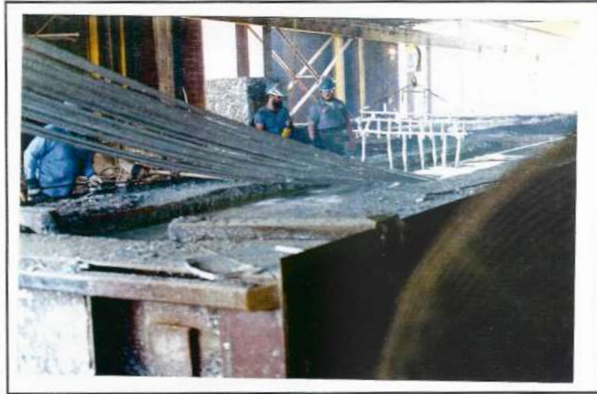
Photo 7 Reinforcing steel being galvanized. Material longer than the zinc bath can be galvanized by dipping one half of the material, then dipping the other half.
