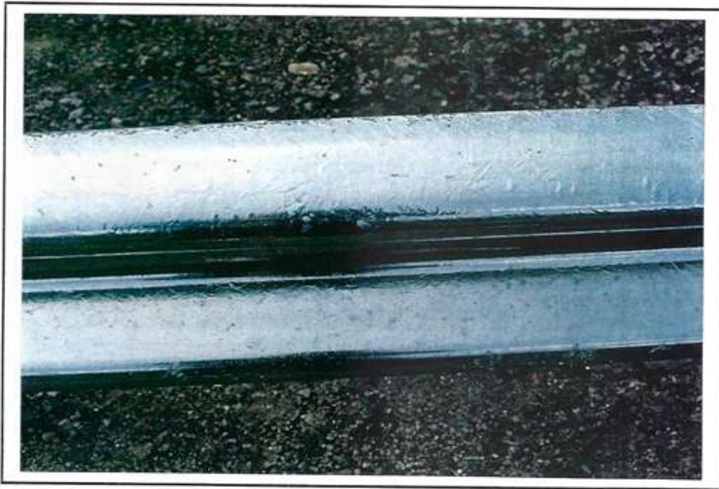
Photo 32 Condition: General Roughness
