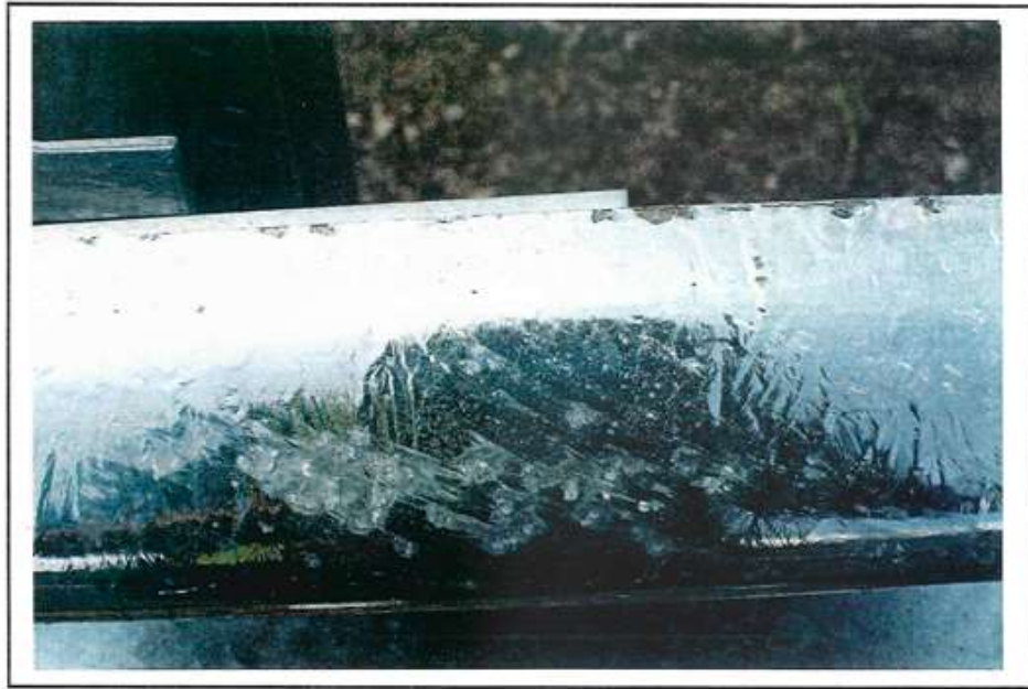
Photo 38 Condition: Bare Spots (Exposed Steel)
