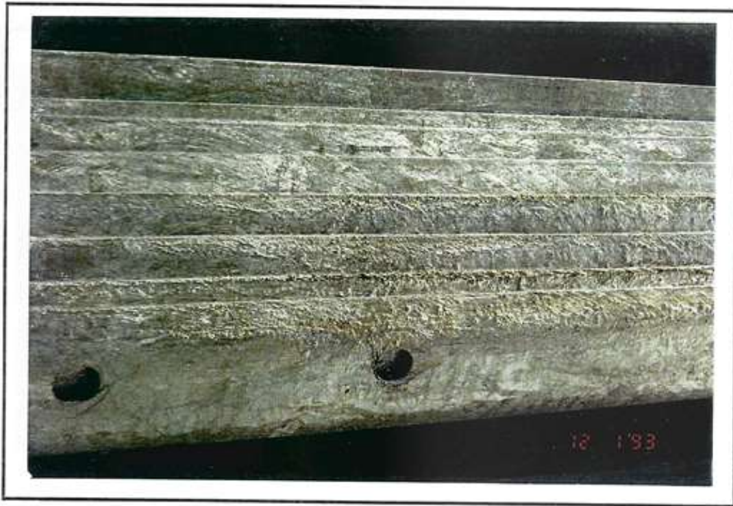
Photo 34 Condition: General Roughness
