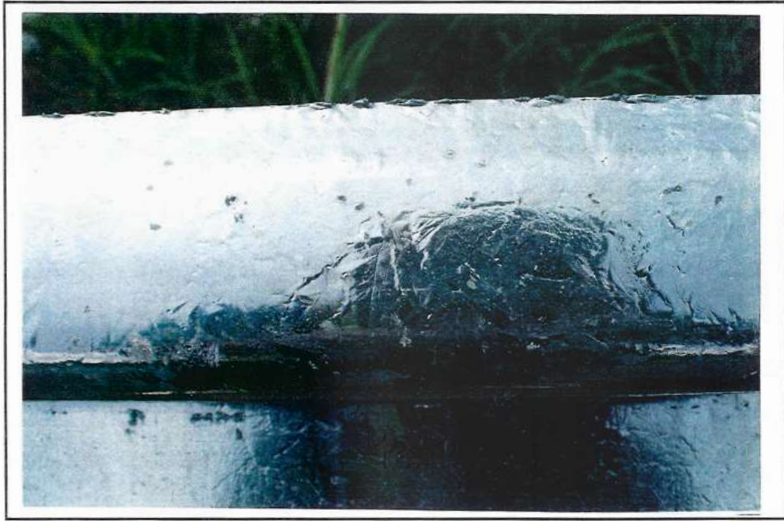
Photo 30 Condition: General Roughness
