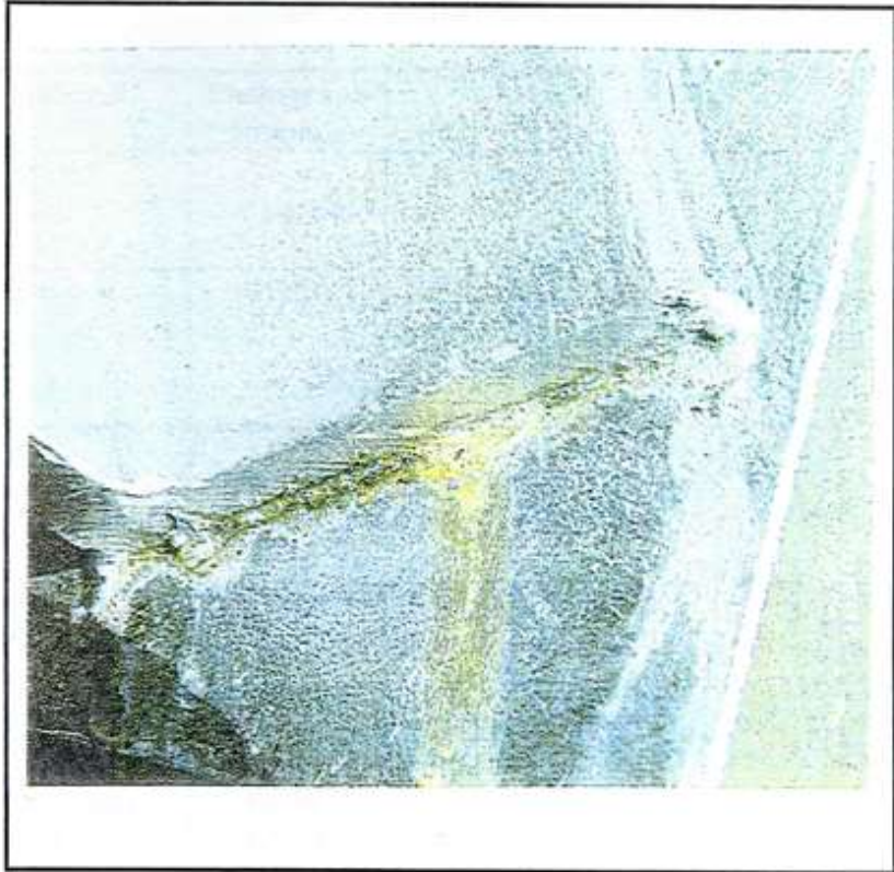
Photo 36 Condition: Rust Stain Caused by Seepage
