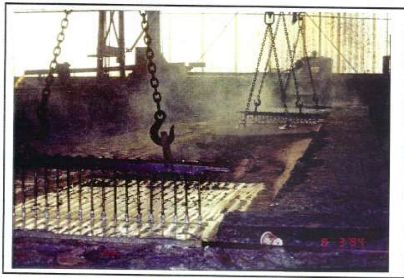
Photo 8 Guardrail material in zinc bath. Notice the ash has already returned to the surface of zinc. This must be removed before the material is removed from bath or it will stick to the guardrail.
