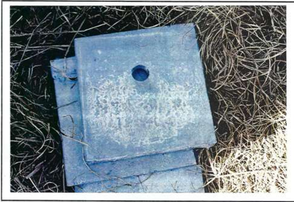
Photo 74 Condition: Wet Storage Stains (White Rust)
