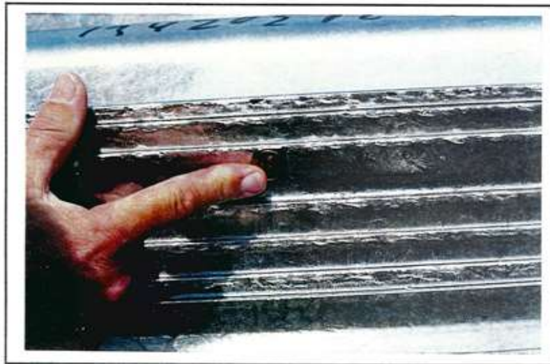
Photo 46 Condition: Bare spots on edge of guardrail. Cause: Breaking off of excess material.
