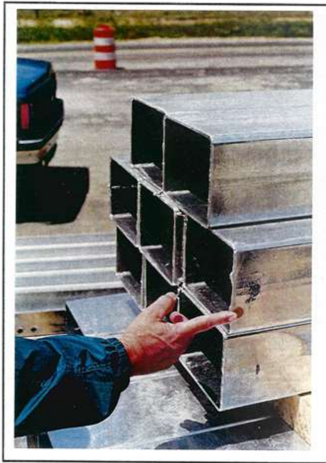
Photo 41 Condition: Bare Spots (Ungalvanized Areas)
