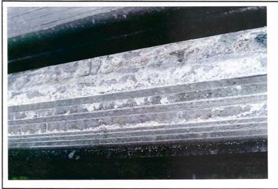
Photo 72 Condition: Wet Storage Stains (White Rust)
